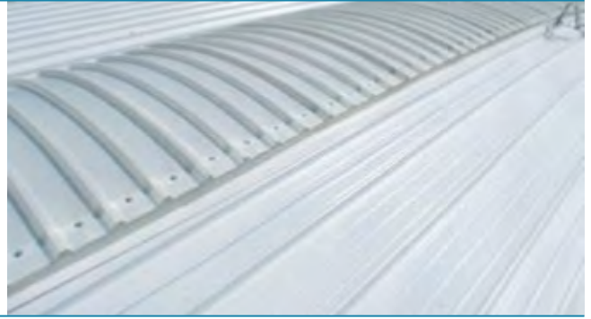
GRP barrel vault
